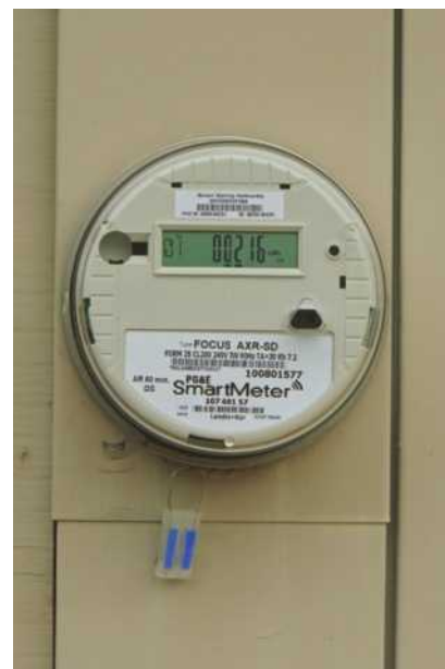
Figure 7.31 Modern, digital smart meter equipped with a radio frequency transmitter and capable of providing automated meter reading (as well as other services) as part of local monitoring network.
